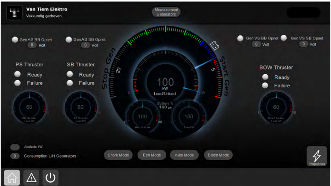
Utilizing Power Management System
